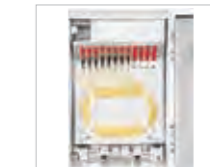
Indoor optical fiber cable distribution box
