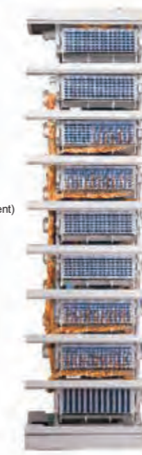
On side of external trunk cable
