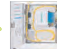
Optical cable splitter in passageway
