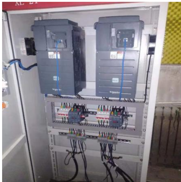
Variable-Frequency Cooling Pump
