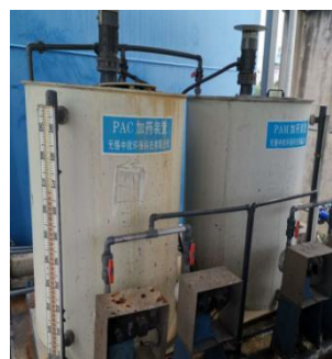
automatic dosing devices
