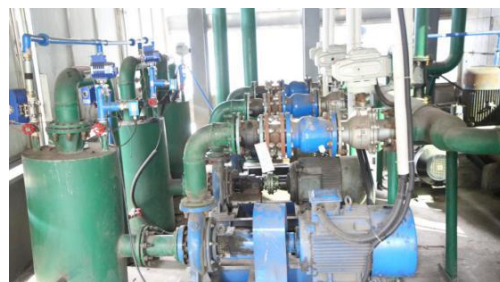
Centralized refrigeration by cooling tower
