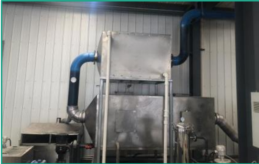
Disposal for high temperature waste gas
