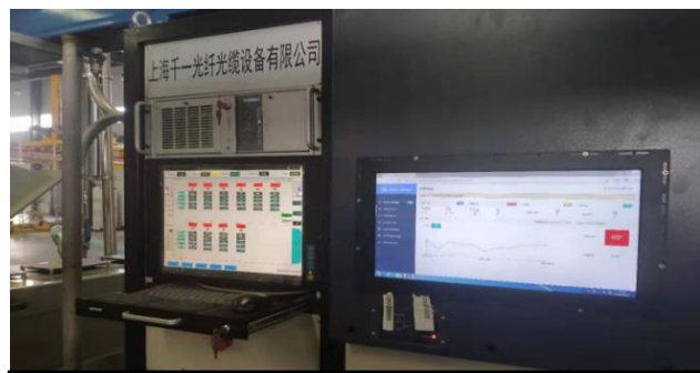
intelligent machine information terminal system
